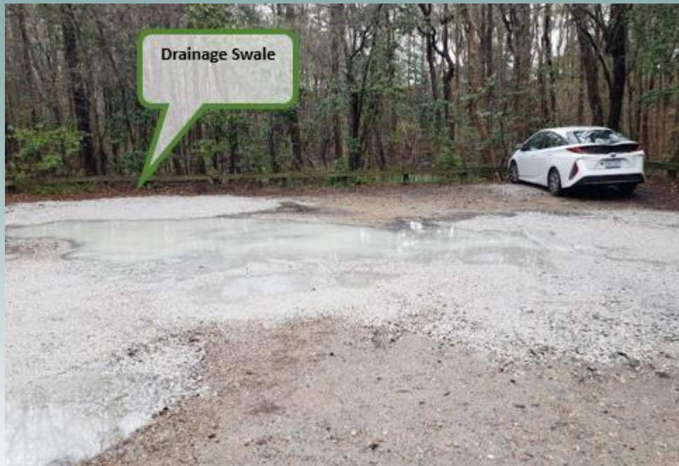
64 th St. after heavy rain of March 22. Puddle issues improved with gravel & drainage swale.
